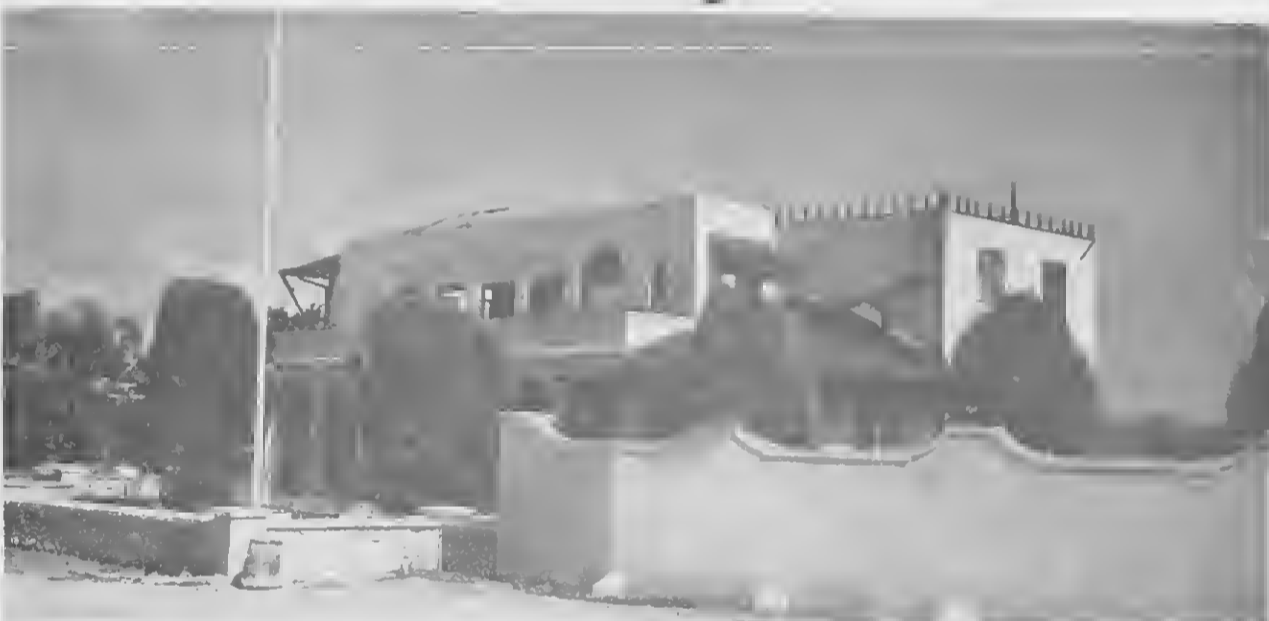
THE END of an era came to pass recently with the demolition of Casa Grande. The 15-room home, which overlooked Lone Palm Stadium and the Baby Lagoon, was built for L. G. Smith in May, 1934.
